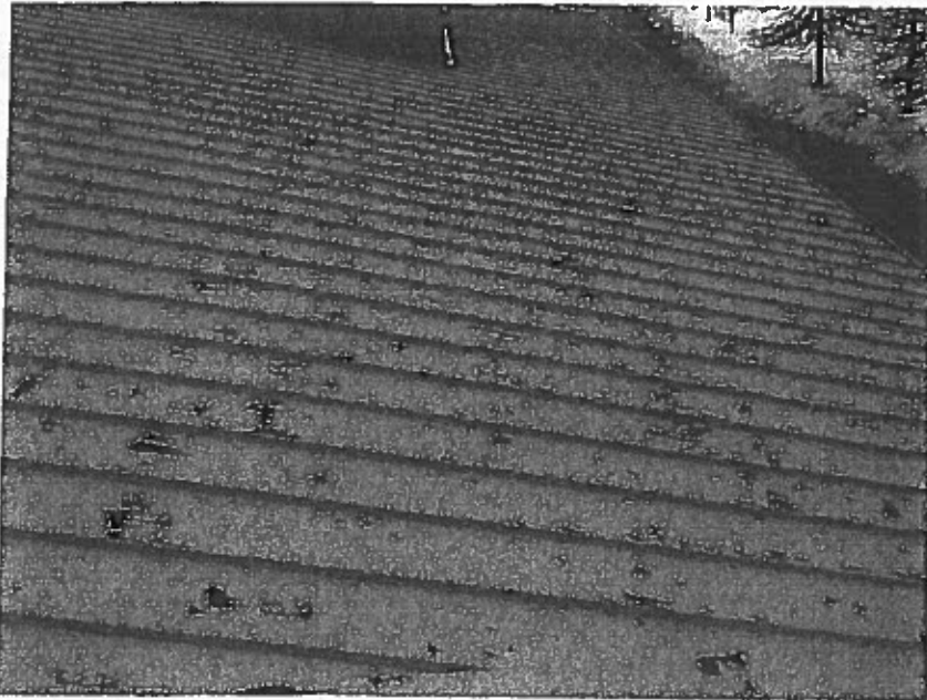
The spot rusting needs to be addressed prior to a full roof replacement being necessary.
